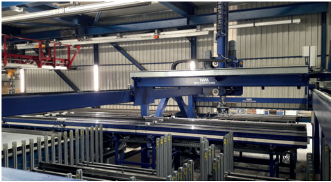
The new magazine robot with the expanded magazine and new cycling roller conveyors
