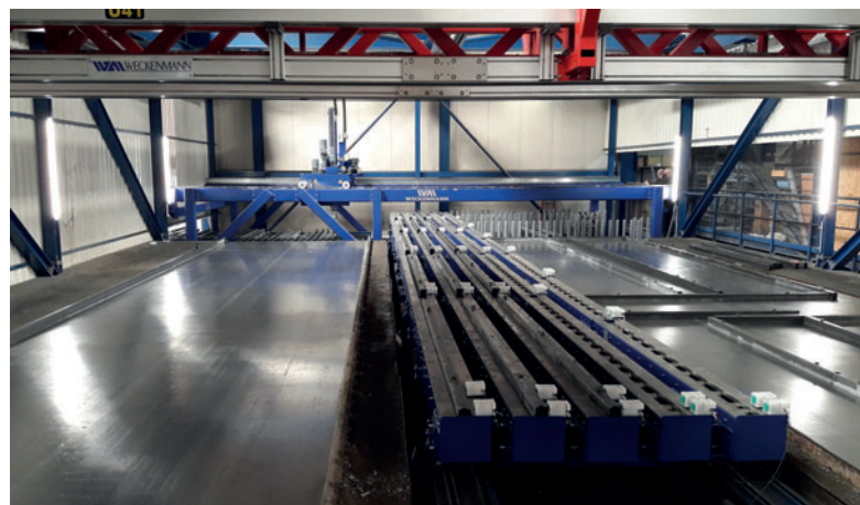
After modernisation: Formwork plant with new cycling roller conveyor and new Weckenmann magazine robot
